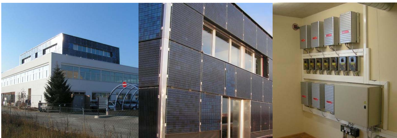
Figure 5 Photovoltaic cladding system and building services control room with grid-tied supply switching system, designed and installed by ATB Becker, Absam, Austria.
